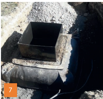
7 The chamber grounding process.
