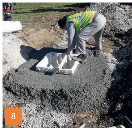
8 Preparation and concrete foundation levelling for the RC ring with a cast iron cover.
